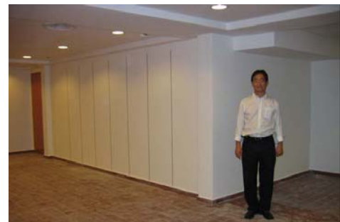
Pilot test using low-cost lightweight wall panels, produced in lab and erected on site in June 2005 at the Centre for the Arts at NUS.
