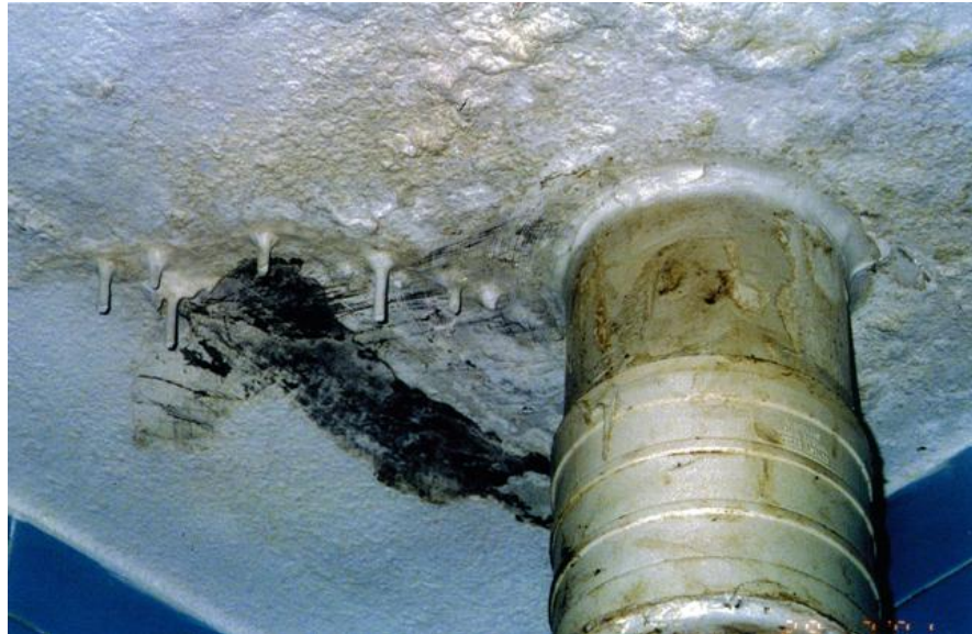
Figure 1: Typical Toilet Leakage Around Floor Pipes
