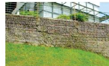
Before repair: Cracked earth retaining wall
