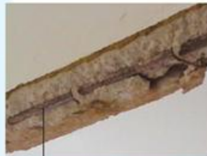
Steel bars corrosion and spalling concrete
