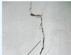
Cracks on beam
