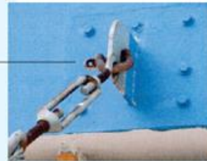
Corroded steel connection
