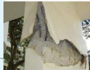
Cracked and spalling concrete on column
