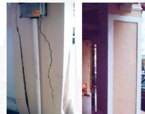
Before: Cracked column
