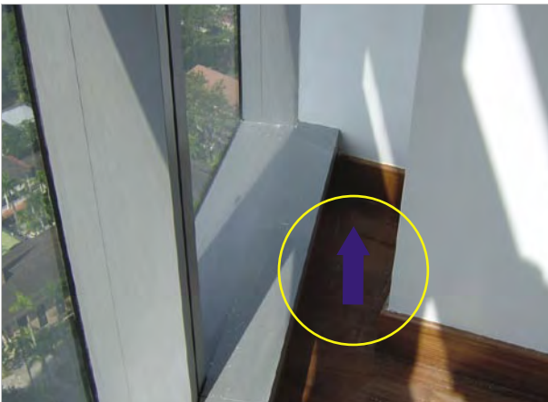
Fig. 2.7 - Small recesses: Difficult to carry out works like skirting, etc.
