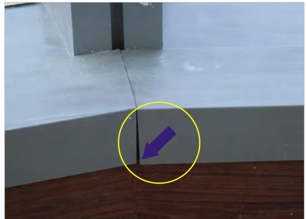
Fig. 2.8 - Protrusions in aluminium capping due to too many jointing segments.
