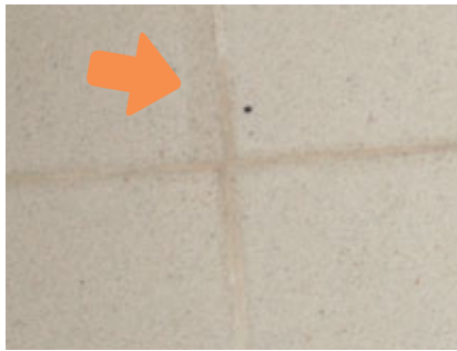
Fig. 6.4 – Discoloration of grout and edge staining after polishing.
