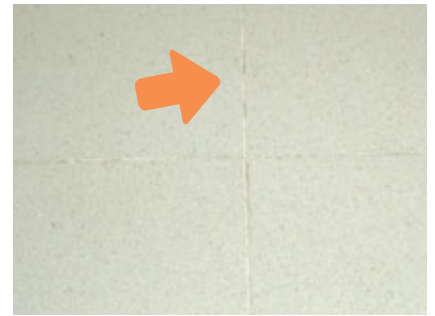
Fig. 6.5 – Emerging grouts from marble joints.
